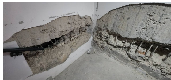
Figure 1. Concrete Crushing in RC Wall of a 25-Story Building in Bangkok
