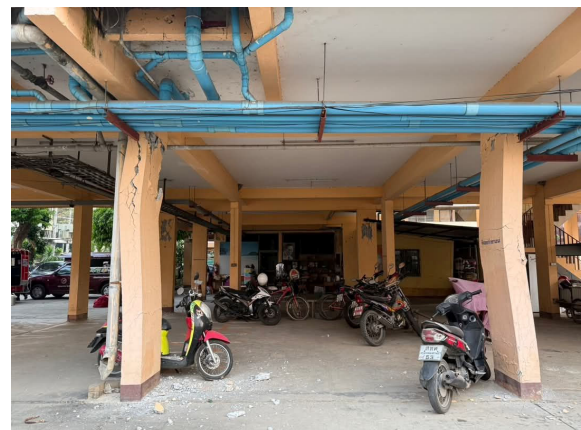
Figure 2. Column Buckling in an 8-Story Building in Chiangmai
