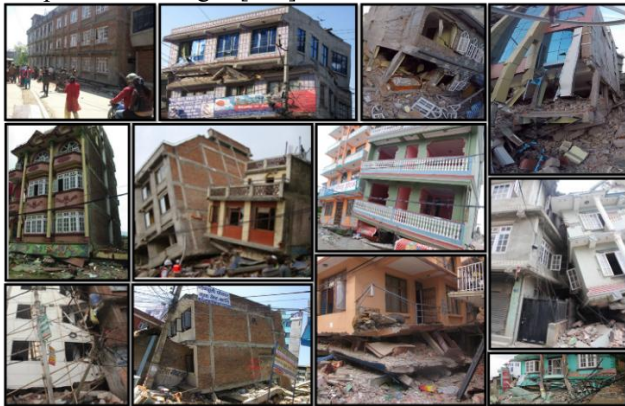
Figure 1. Soft-storey collapses observed in the 2015 Gorkha Earthquake in Nepal
