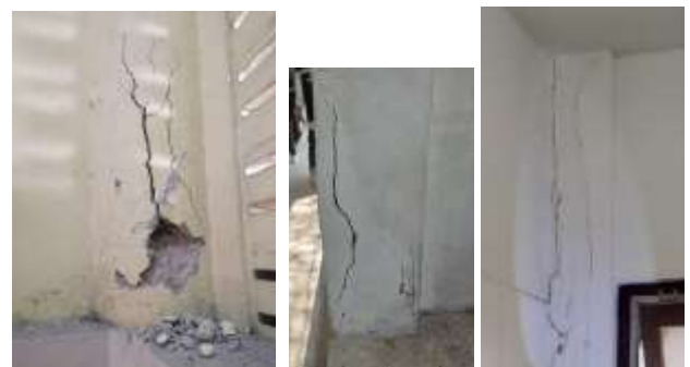
Moderate Damage and Severe Damage
