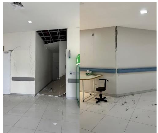
Figure 2. Damaged hospital buildings
